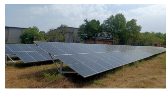
PECIN photovoltaic power generation systems
