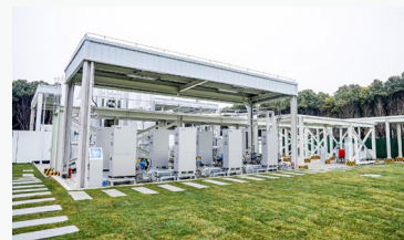
Pure hydrogen fuel cells installed at PECW
