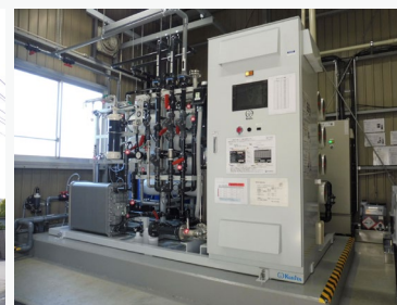
Water purification system with electrical resin regenerator
