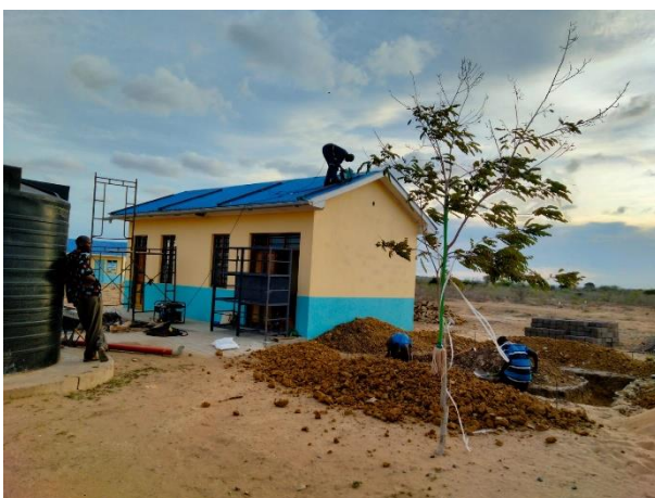
Solar panels on the roof of the maternity ward, with building construction for the PSS in front.
