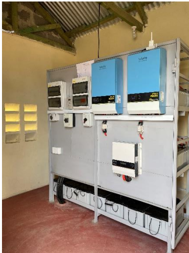
Inside of PSS building with battery and panels installed.
