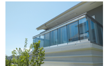
"Energy-generating glass" in harmony with the town and everyday life installed at a model house at Fujisawa SST for demonstration test
