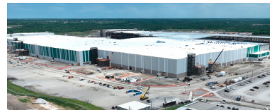
Building our Kansas Factory for more EV battery production capacity (as of April 2024)
