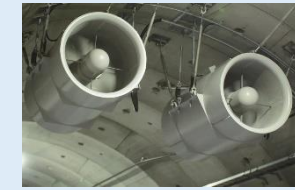
Tunnel ventilation and purification systems
