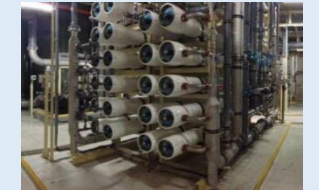
Water treatment systems
