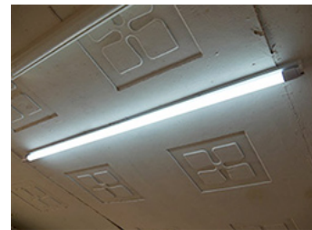
LED lights are installed in the primary school classrooms.
