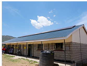
Solar panels installed on the roof of the schoolhouse are now generating power.
