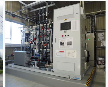
Water purification system with electrical resin regenerator
