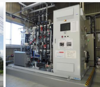
Water purification system with electrical resin regenerator
